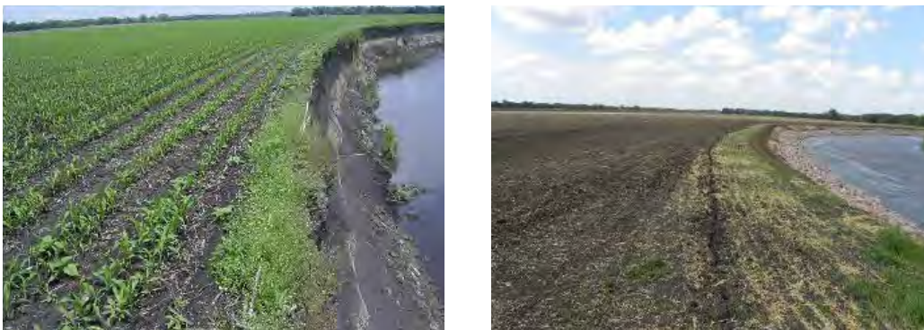
Figure 1. Before and after pictures of a bank stabilization effort along the Big Sioux River near Sioux Falls (EDWDD 2012 4 ).
